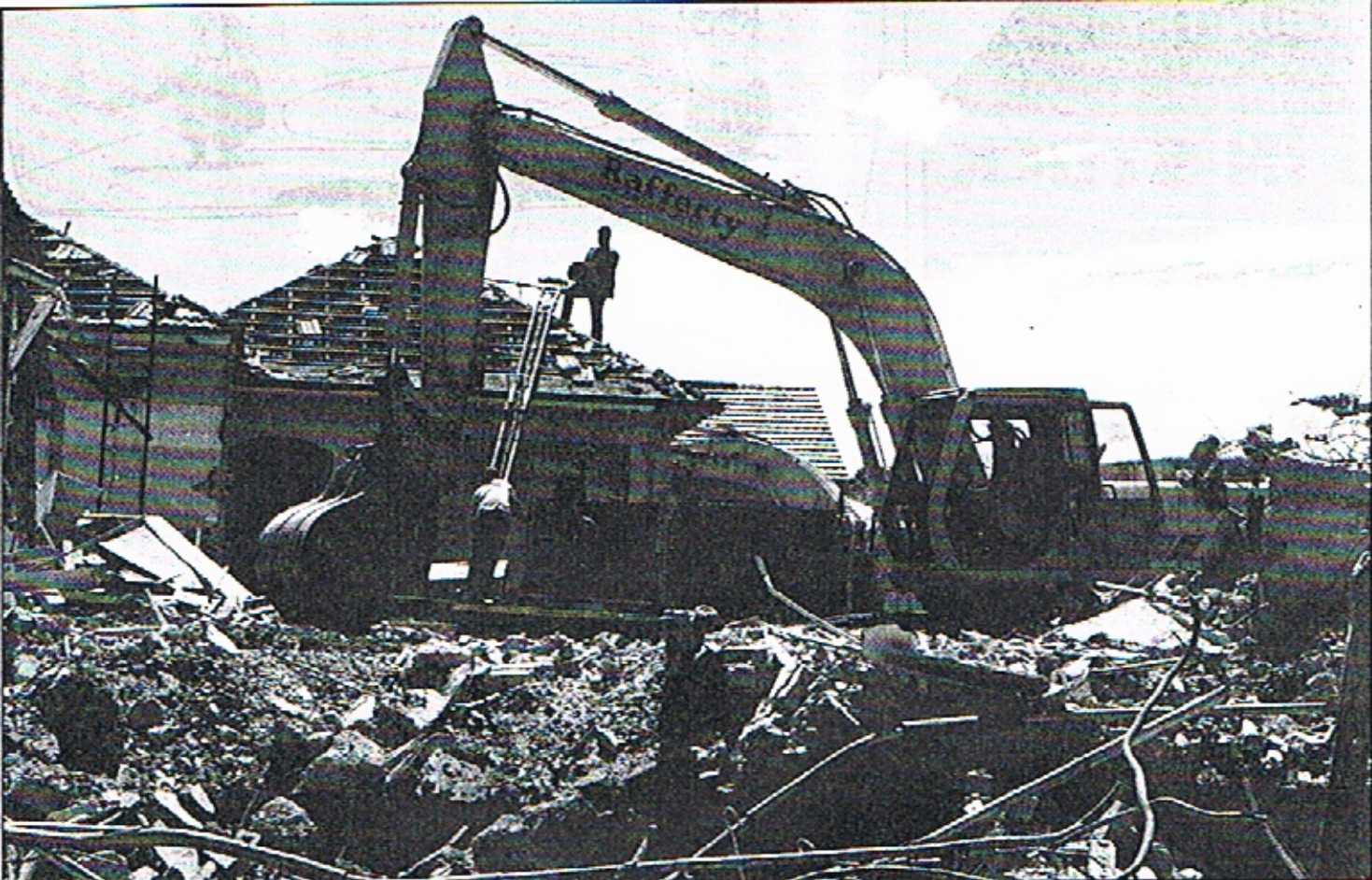
Down it comes: Demolishers arrived at the historically significant house Rothesay to begin work recently, sparking concern among the community and development watchdog groups. The house's owners, Anglican Homes for the Elderly, would not be drawn on their plans for the site. Picture: Peter Weaving
